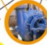
Warman mill circuit pumps
